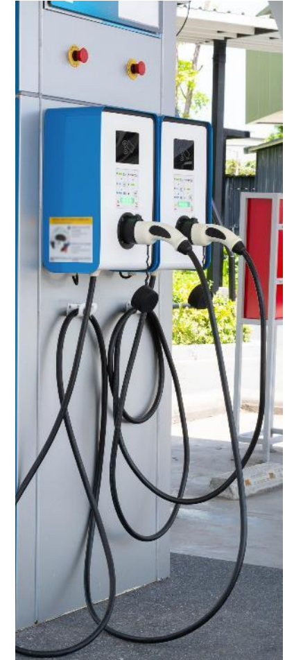
EV charging infrastructure
