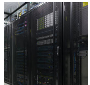
Uninterruptible Power Supply
