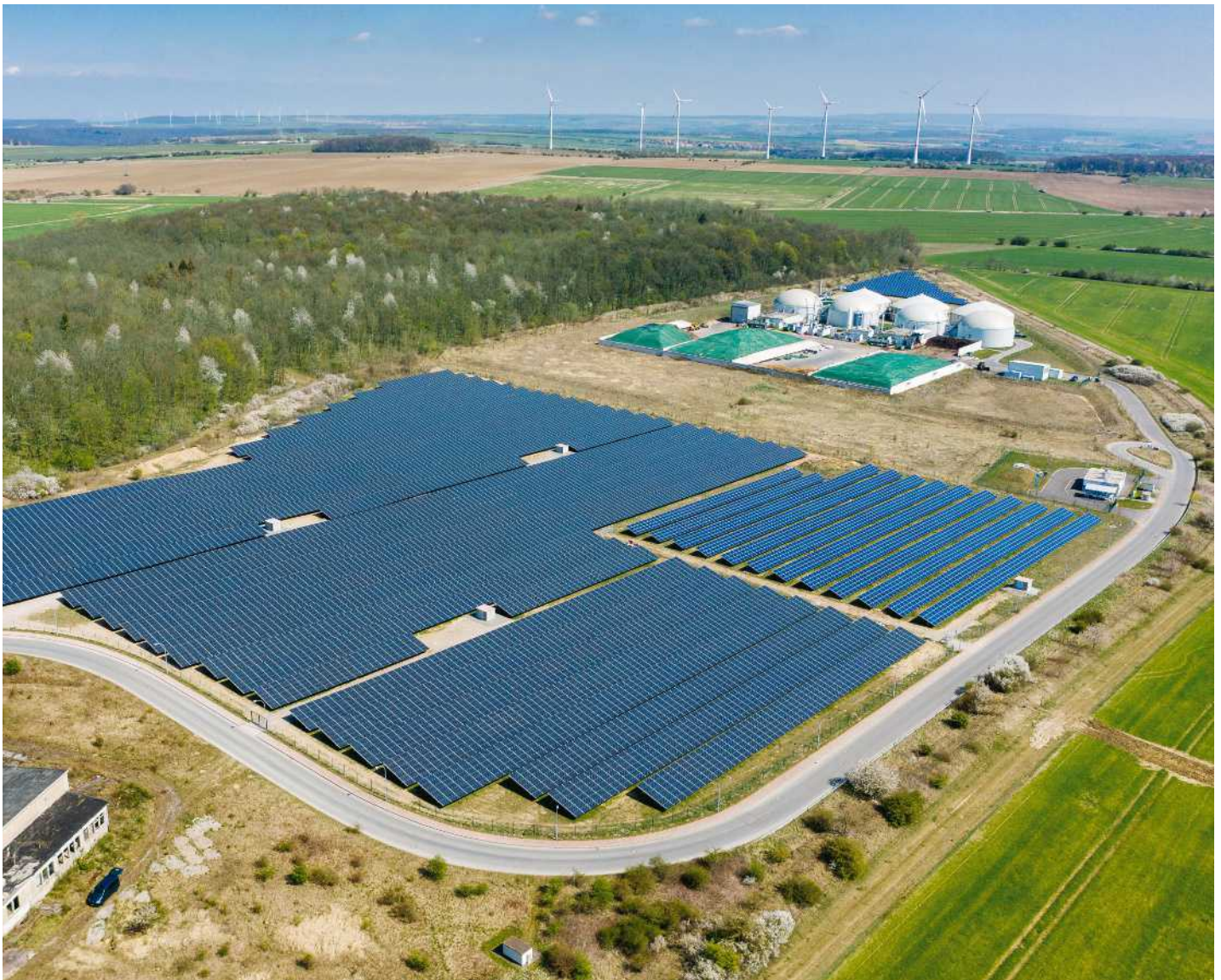
Menteroda solar park, Germany
