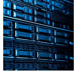
Data Center Server
