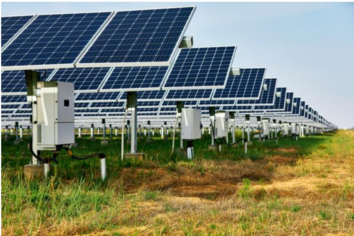
Figure 1. Inverter boxes connected to photovoltaic panels.
