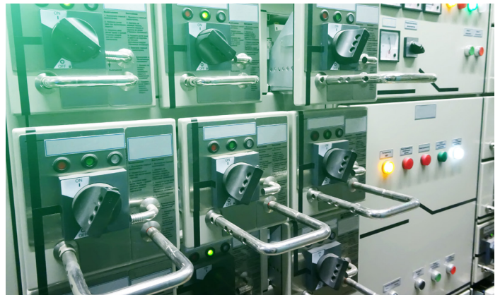
Figure 3. Transformer Substation with Switches and Sensors
