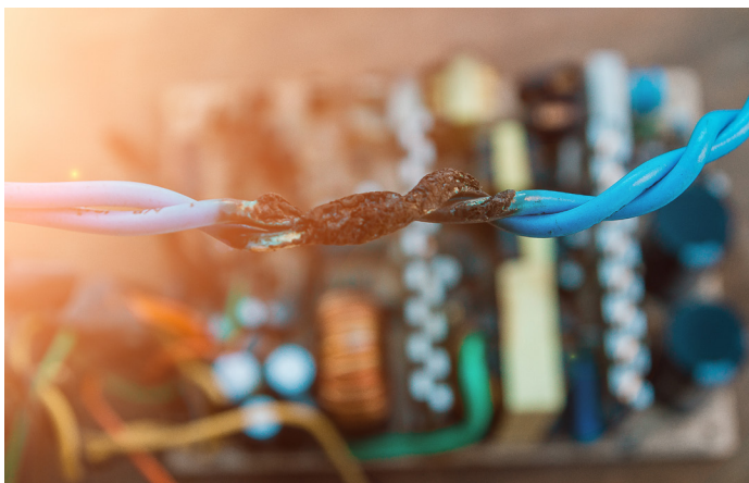
Figure 42. Heat-Damaged Electric Wires - Cable Faults Result in Short-Circuit Faults
