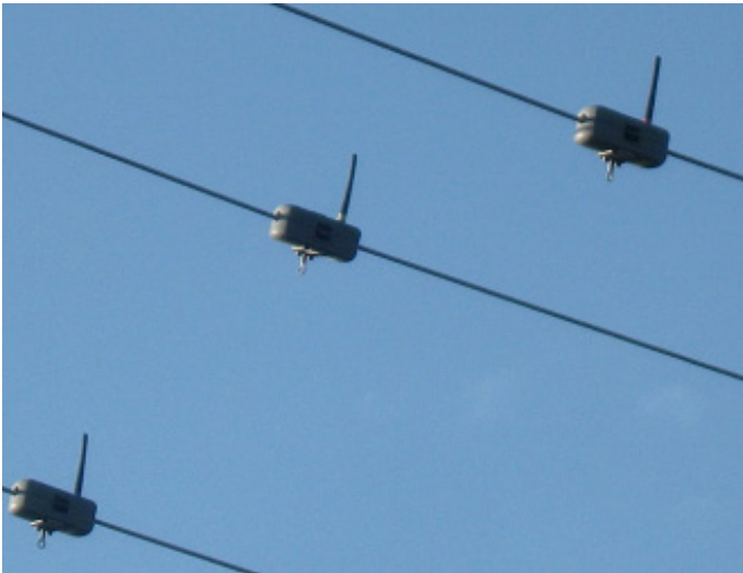
Figure 13. Overhead Line Sensors (Photo licensed under CC BY-SA)
