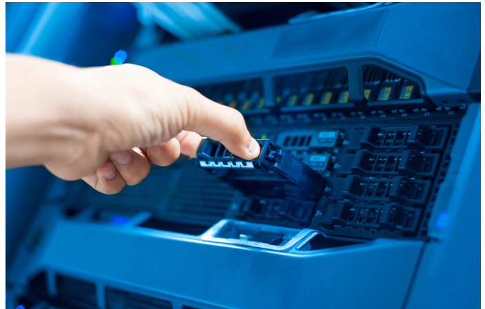
Figure 40. Hot Plug-in Causes Voltage Surges
