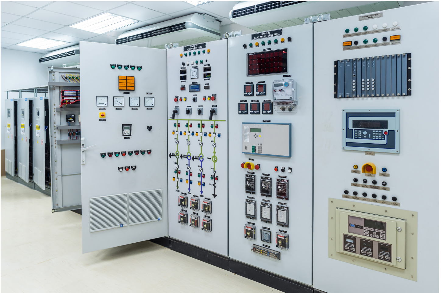
Figure 1. Power Substation Electrical Switchgear
