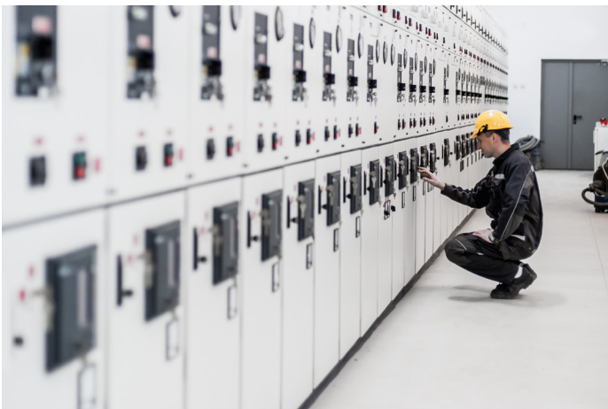
Figure 25. Medium Voltage Switchgear and Bay Control Unit
