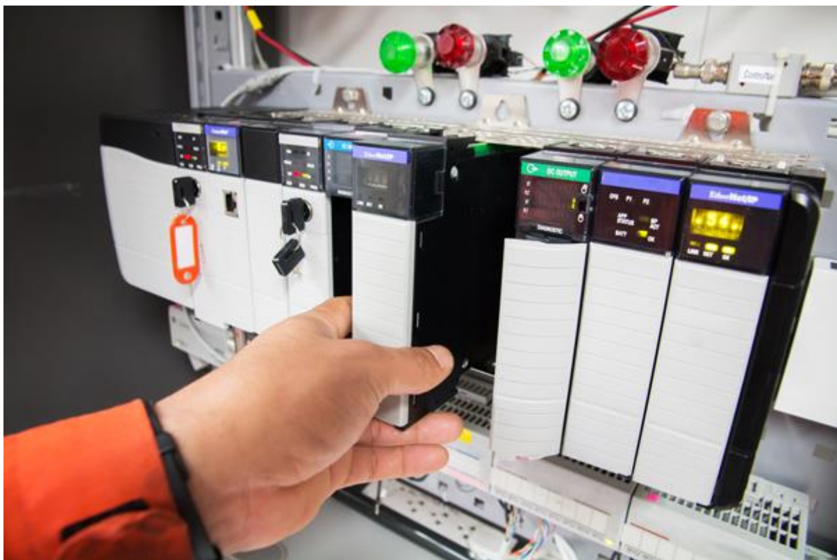
Figure 1. Programmable logic controller module.
