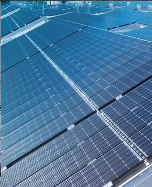
Renewable Energy, Energy Distribution
